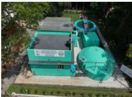
360 KLD STP at General Hospital, Thrissur
