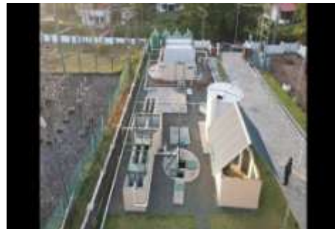
1 MLD CSTP at Padanappalam, Kannur
