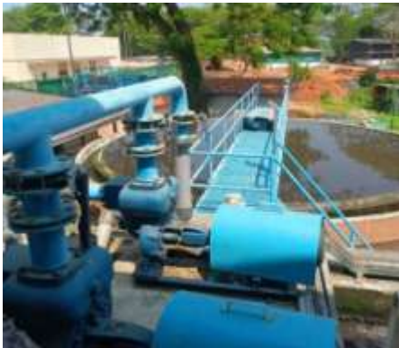
500 KLD STP at Kozhikode medical College
