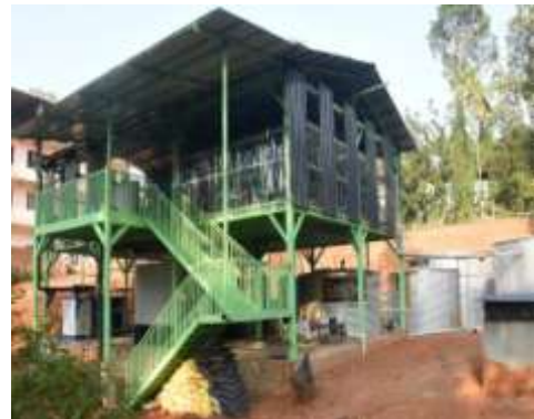
1 MLD STP at Kozhikode medical College
